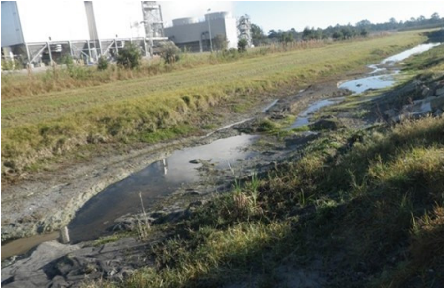
Figure 10. Sediment Accumulation in the Northern Drainage Ditch
