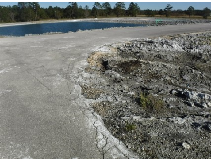
Figure 7. Erosion on the Northern Inside Corner of Ash Cell #2
