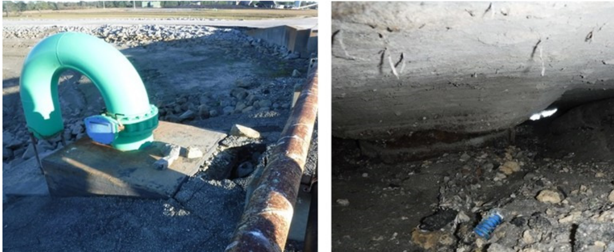
Figure 9. Above- and Below-Grade Conditions of the Southern-Most Splash Block in Ash Cell #2
