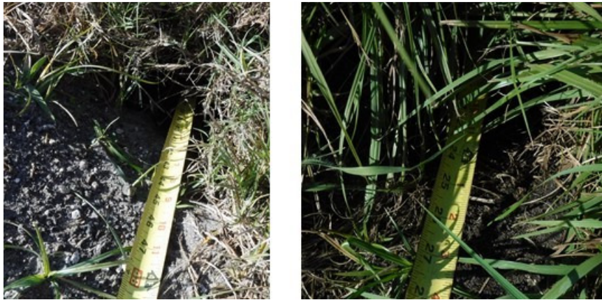
Figure 14. Animal Burrows/Forage Holes and Hole Depths Observed on the Southern Slope of the CCR Landfill
