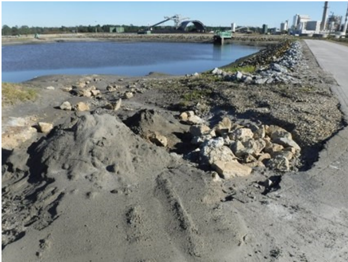
Figure 5. Erosion on the Western Inside Corner of Ash Cell #1
