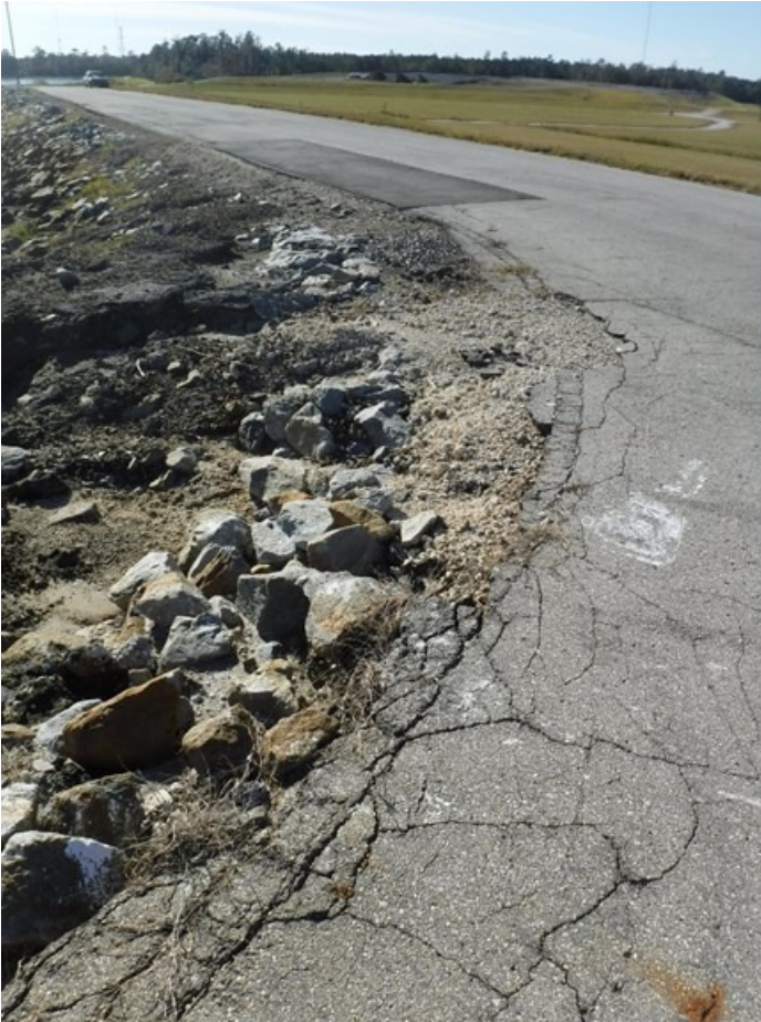
Figure 6. Erosion on the Northern Inside Corner of Ash Cell #1
