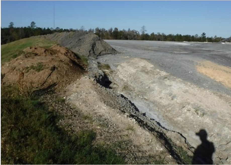
Figure 11. Erosion near Cell 2/Cell 3 Access Ramp
